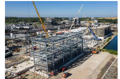
HHCR Hydrogenation Unit
